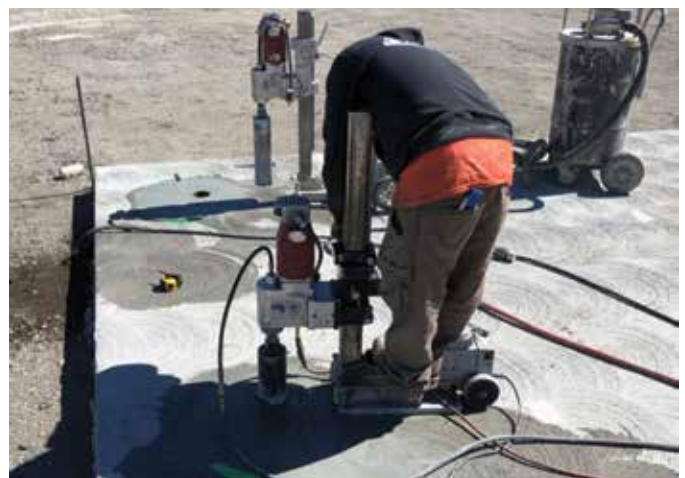
Fig. 5: Two core drilling machines were used to extract the nominal 4 in. diameter cores that were then measured for thickness
