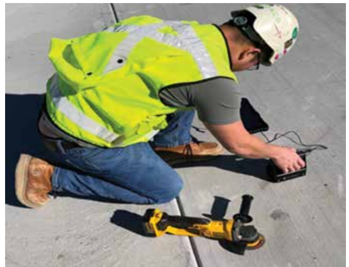
Fig. 4: IE was used to obtain slab thickness at various locations on the concrete surface. As needed, the surface was ground smooth to ensure solid contact with the transducer
