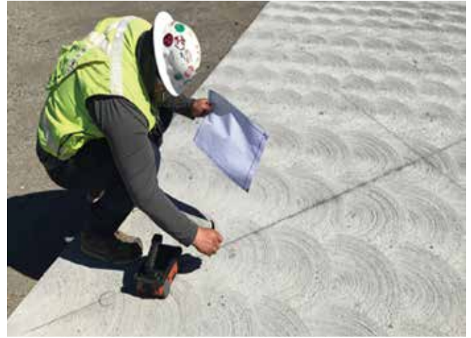
Fig. 3: GPR was used to obtain slab thickness at different locations on the concrete surface
